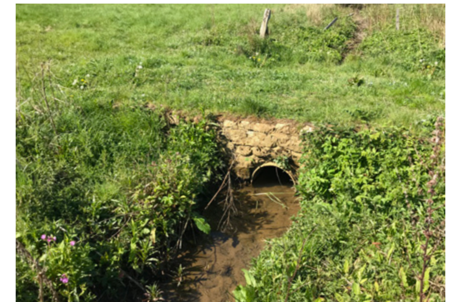
Plastic pipe culvert with stone ends in the middle of the stream.
