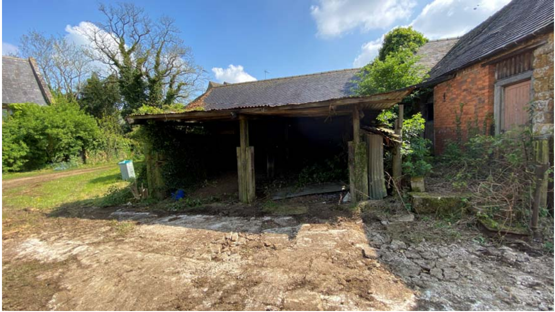
Open lean to recommended to be demolished
