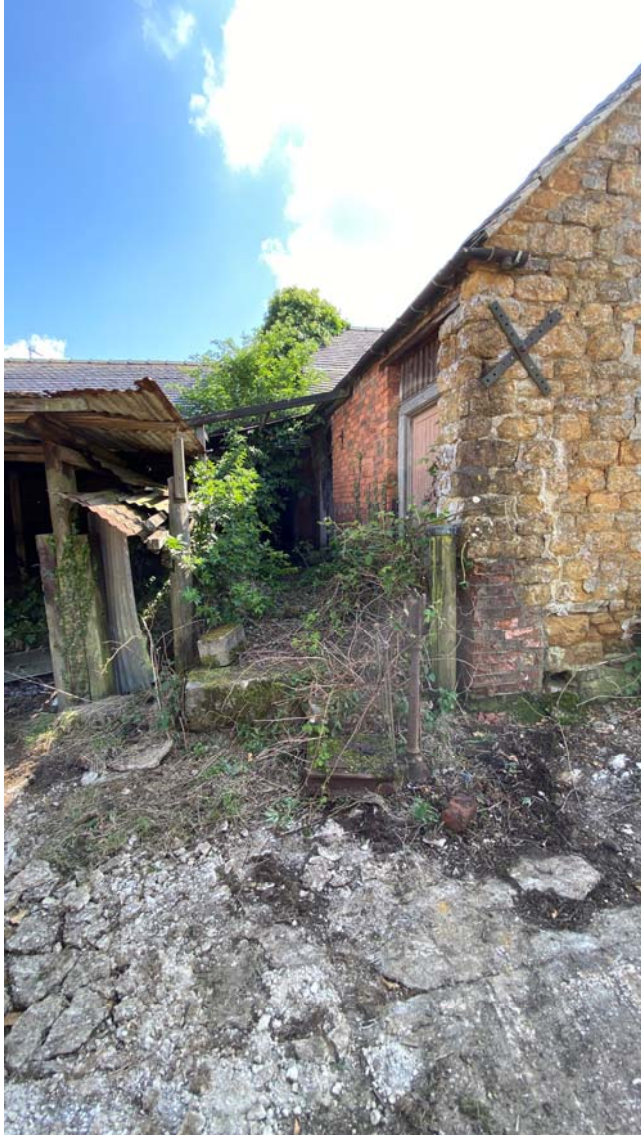
Northern section with mixture of brickwork and stonework. Tie rod and patress visible at eaves
