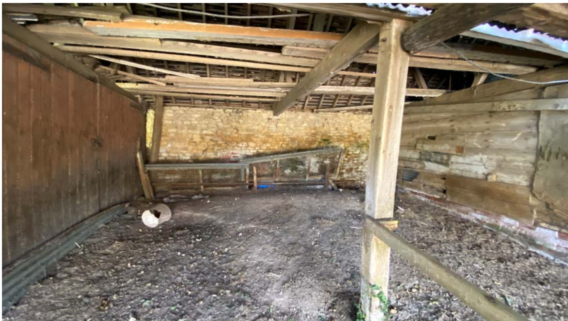
Rear wall of hovel, Some dampness visible from floor to approx mid height
