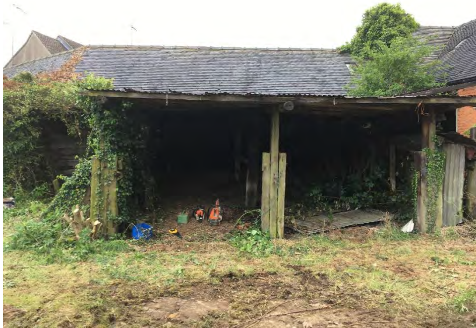
Photo 5: The site south showing the dilapidated farm buildings.
