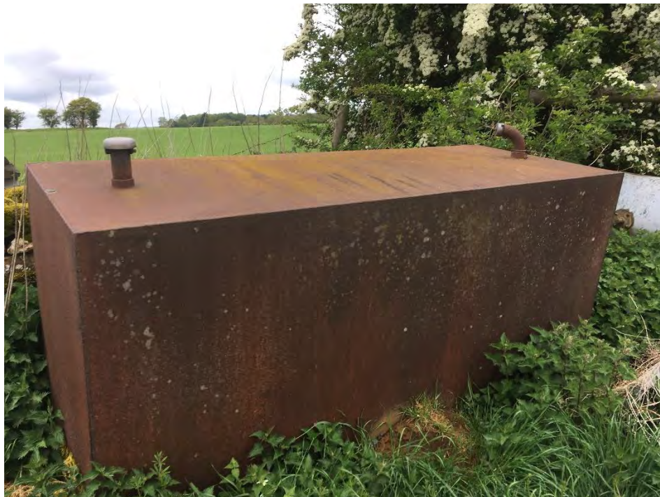
Photo 10: Empty non-bunded metal tank with some obvious rusting and slight pitting located in the neighbouring field.
