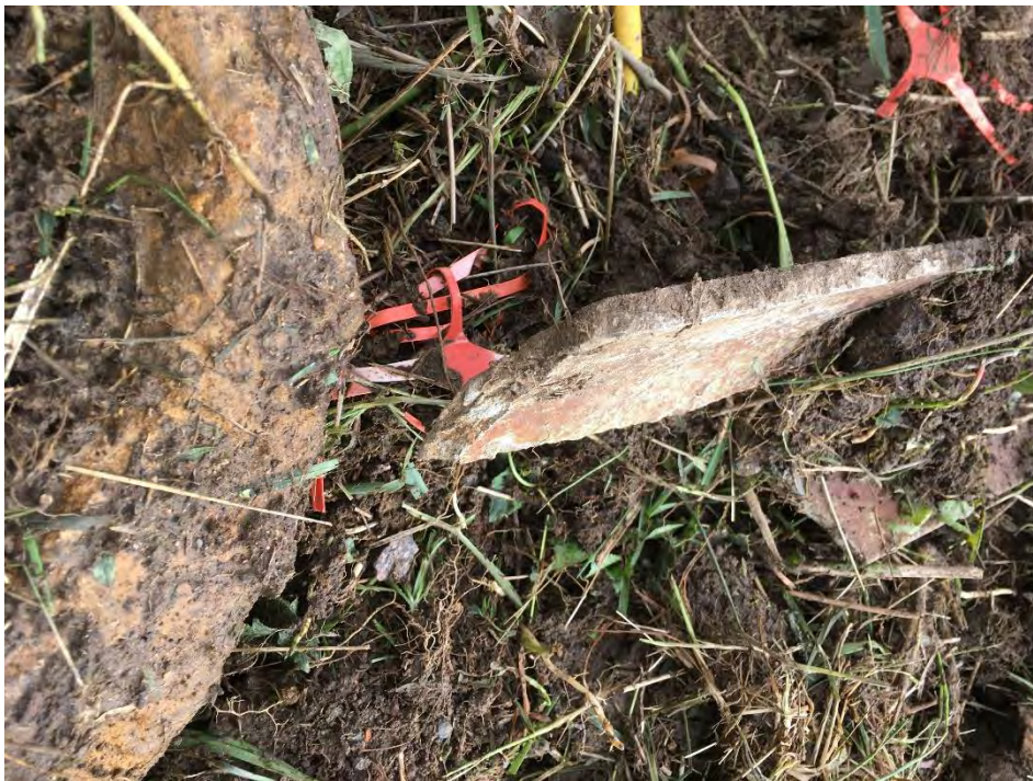
Photo 12: Fragment of suspected asbestos corrugated roofing observed local to TP02 located to the east of the site.
