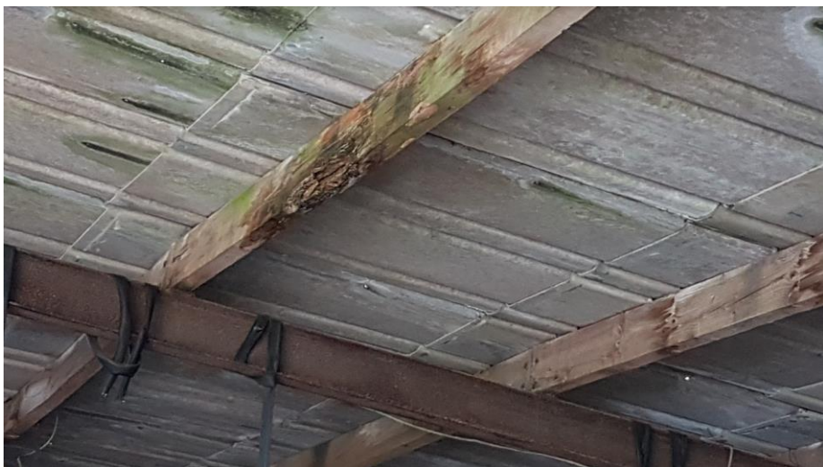
Water damage to purlins
