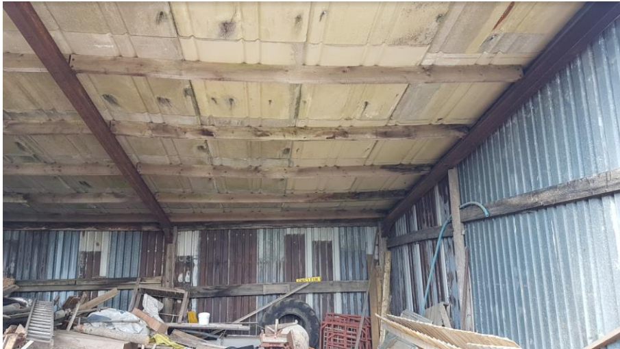
Roof purlins showing sag at midspan
