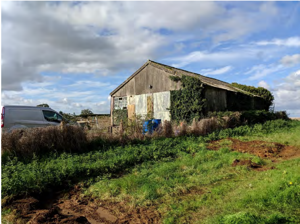
Plate 1: View north west of the existing structure on the site beyond the boundary between Field A and Field B.
