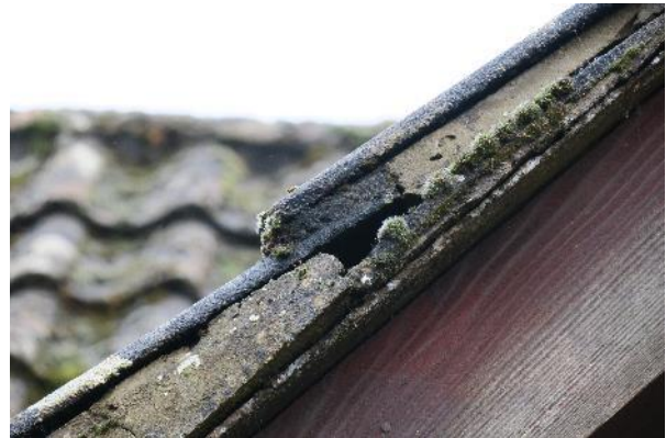
Photograph 10. A gap created by missing mortar at the northern elevation of Building F.
