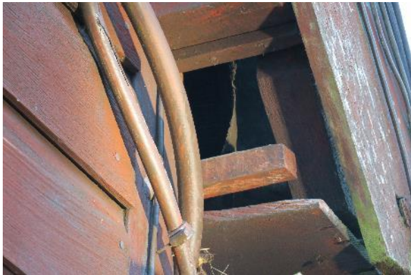
Photograph 9. One of several holes at the eaves of Building F's (northern elevation).
