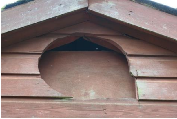
Photograph 7. Partially boarded up hole in northern elevation of Building D.
