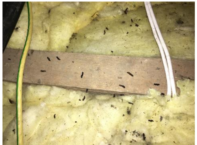
Photograph 4. Accumulation of bat droppings within Building F's loft void
