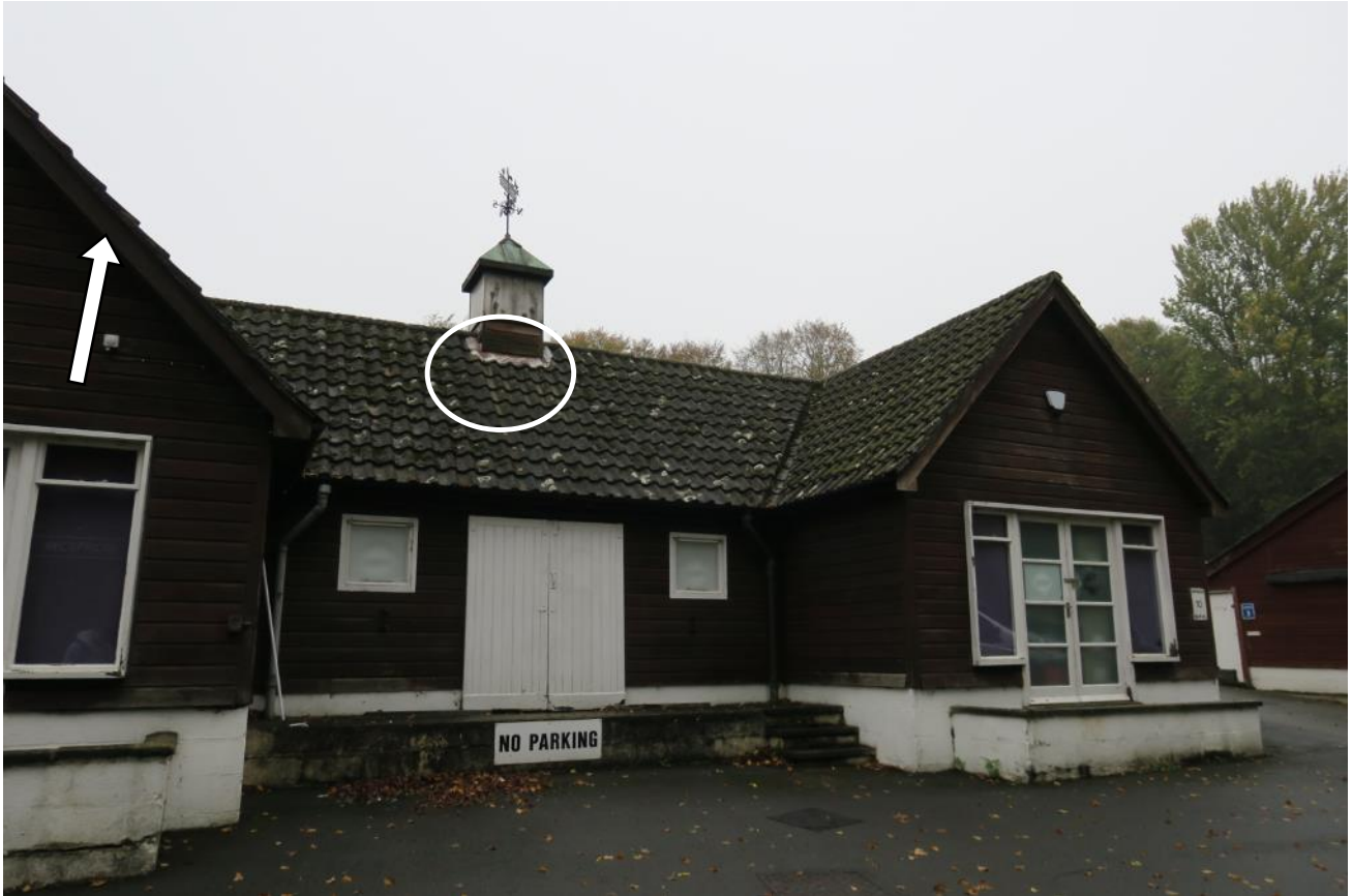
Figure 3. Photograph showing Building F, viewed from the east. White arrow indicates boxed eaves from which soprano pipistrelles were seen to emerge during three bat activity surveys. White circle indicates approximate area of roof from which brown long-eared bats were seen to emerge on the 15/08/19 & 03/09/19.
