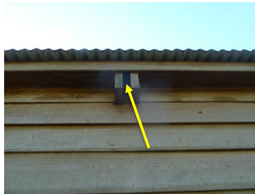
Photo 7: Potential bat access to interior of building 3
