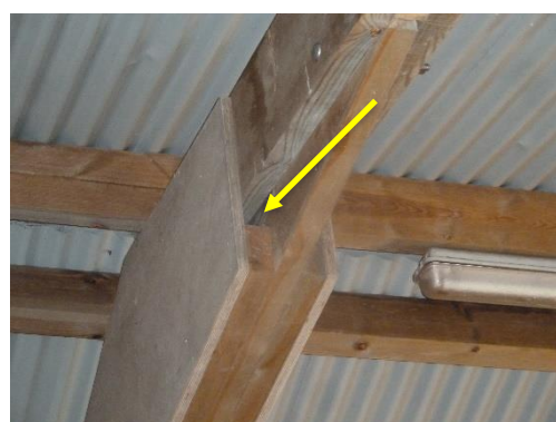
Photo 9: Plyboard 'baffle' at ridgeboard, full of cobwebs
