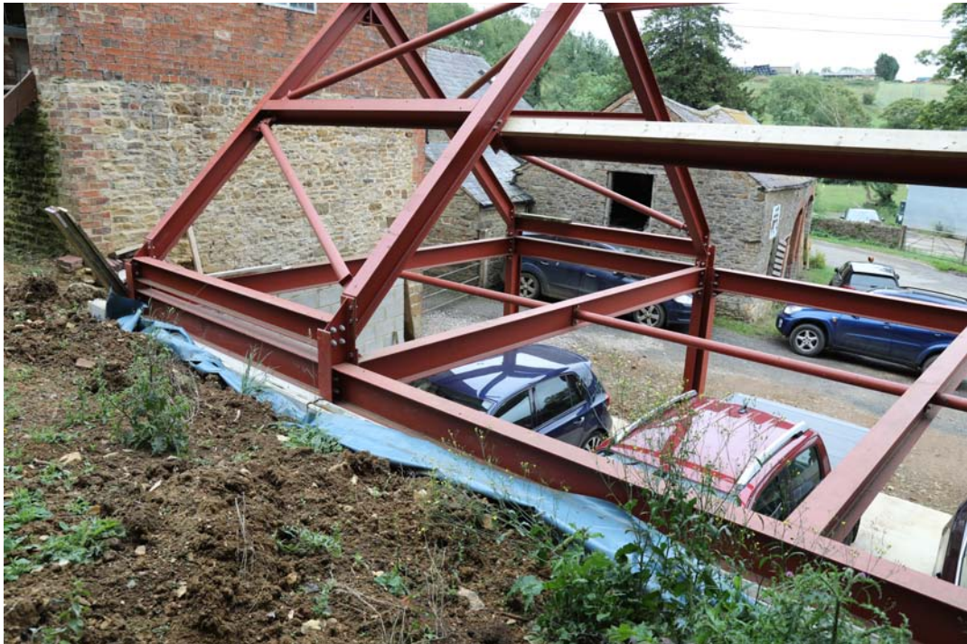
Photograph 3: The rear of the structure from atop the 3m high earth bank
