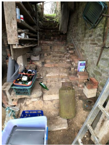
Photo 5: the delapidated brick steps
