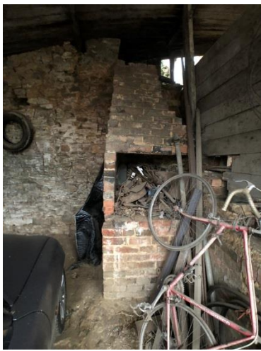
Photo 4: the delapidated furnace to the back of the lean to car port
