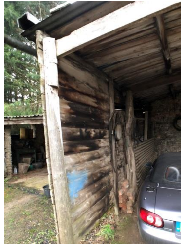
Photo 6: the delapidated lean to structure
