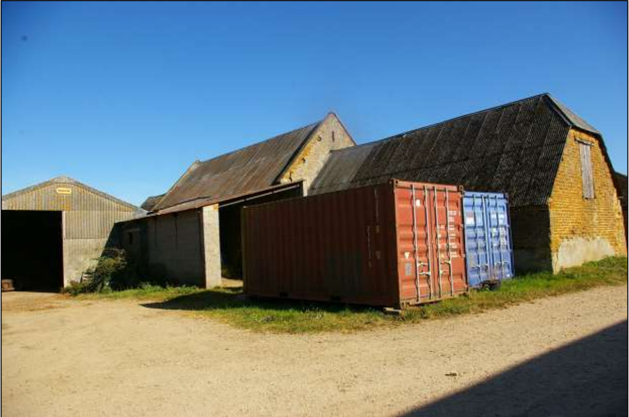
VIEW SHOWING THE MODERN SHEDS THAT ABUT AND ENCLOSE THE HISTORIC THRESHING BARN ON ITS NORTH SIDE; VIEWED FROM THE WEST-NORTH-WEST.
