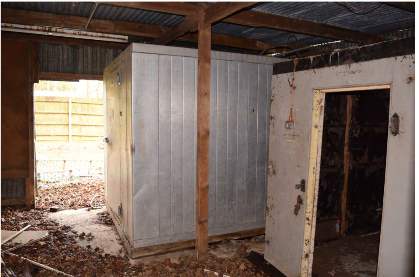
Plate 457.22 View of refrigeration unit store
