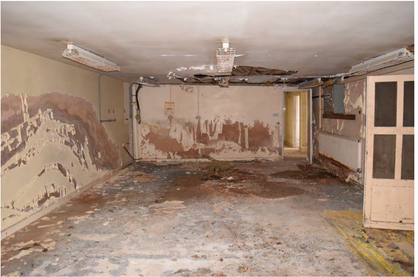
Plate 457.21 View of cold store
