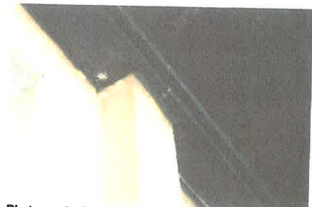
Photograph 4. A gap at the eaves of the western elevation.
