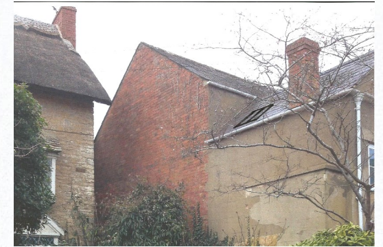
Photograph showing location of new roof window to be installed into existing slated roof
