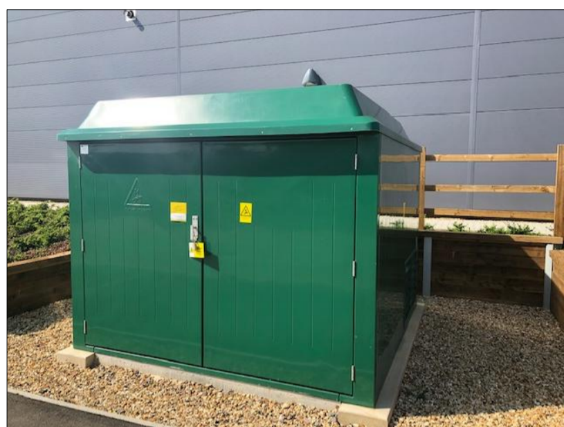
Sub station elsewhere on site.
