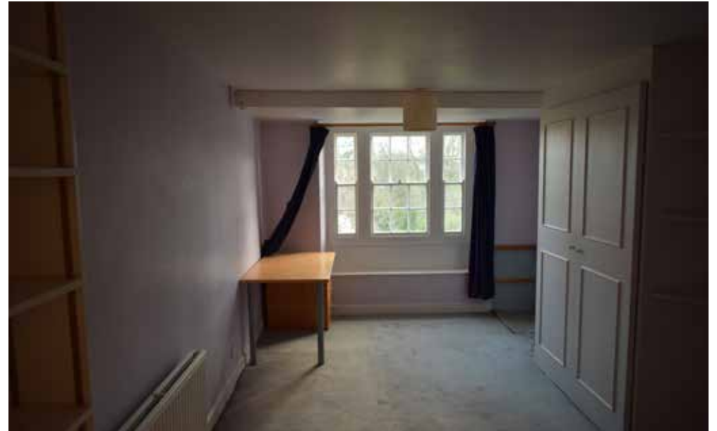
Fig A3.4: Small box room extended c. 1930s by a lean-to extension over a ground floor bay window. Original size of the room marked by encased ceiling beam. The non-structural partition will create a home office at the window end
