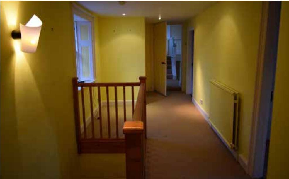
Fig A3.3: Balustrade of the current stair (recent) removed and new balustrade installed. The compliant staircase will land just under the window.
