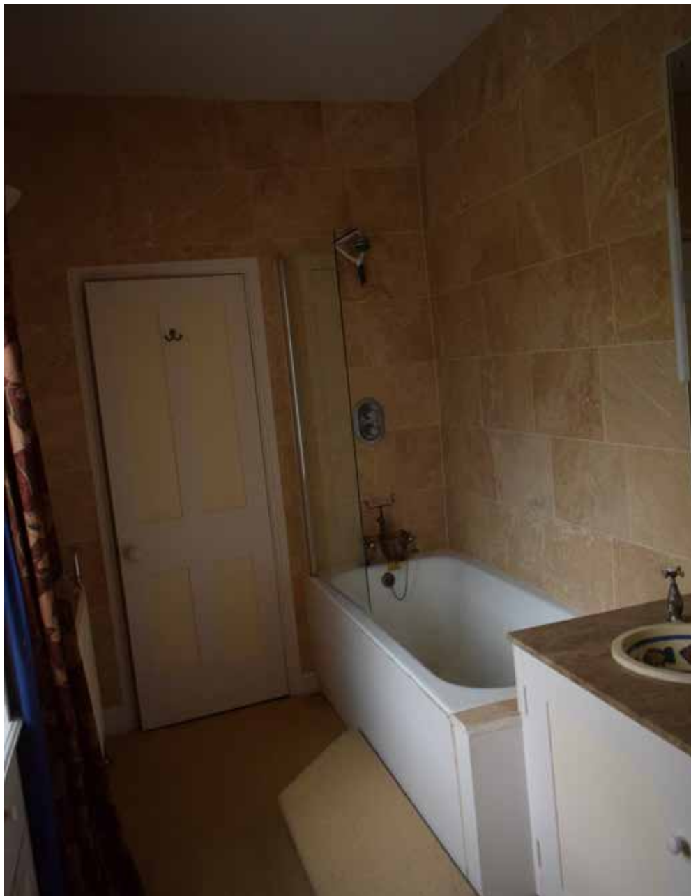
Fig A3.5: View of the ensuite to the Master bedroom. Non-structural wall to toilet to be removed.
