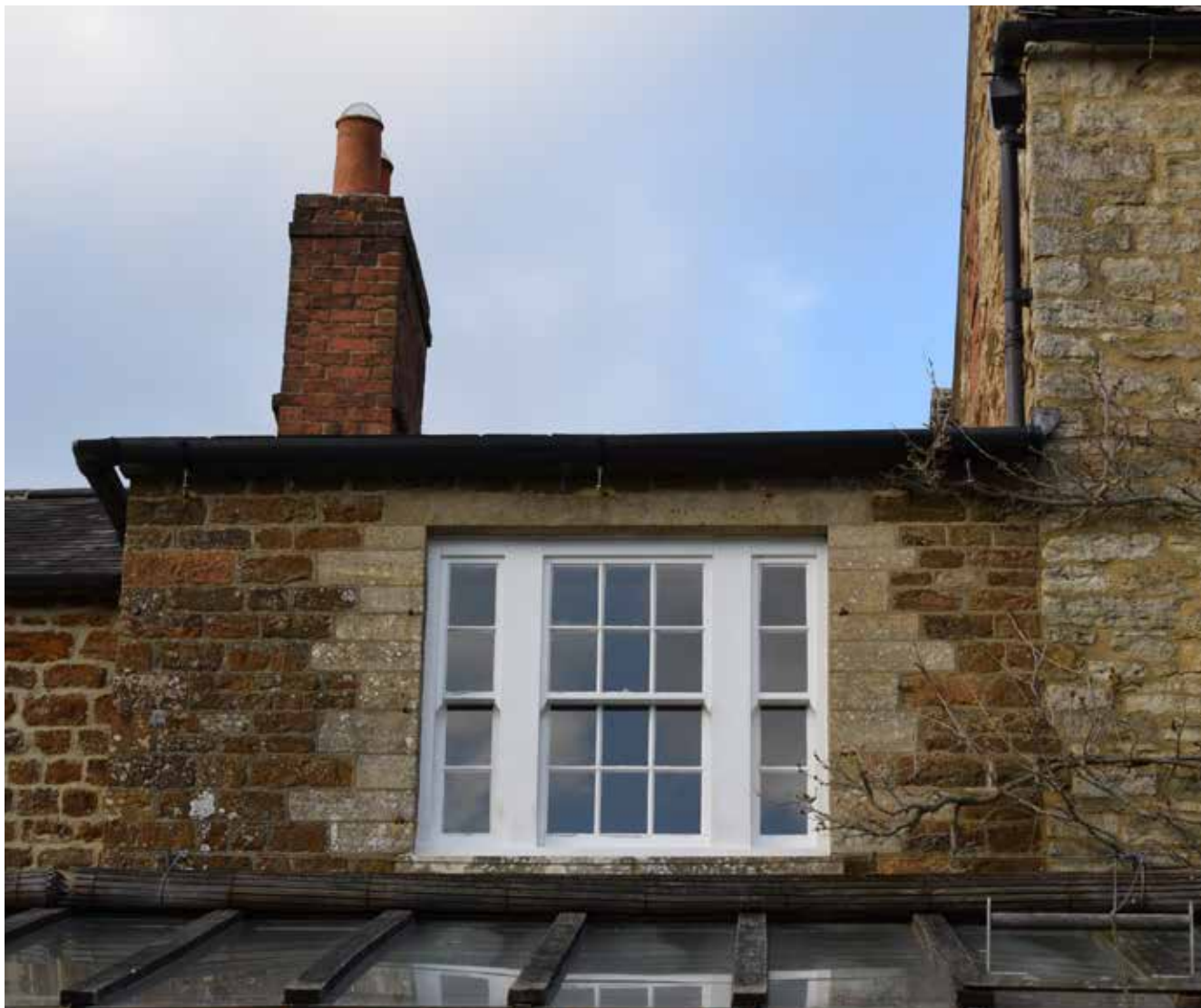
Fig 37: Close up of the tripartite window on the rear (south) elevation of Cedar Lodge for the small box bedroom illustrating the external 'gentrification' of this part of the building to match the window pattern of the main range
