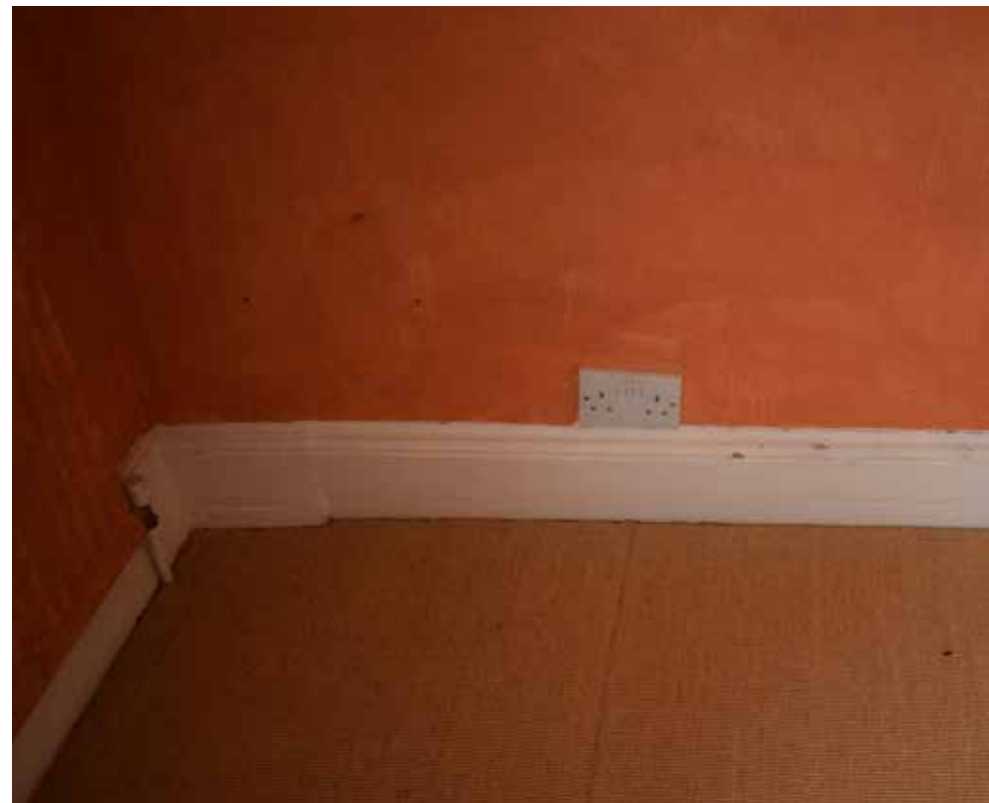
Fig 36: Close-up of the skirting board showing the later inserted piece matching the location and width of the door opening in the other bedroom. Clear evidence there was a door to a shared room at the southern end of the landing lit by the round window
