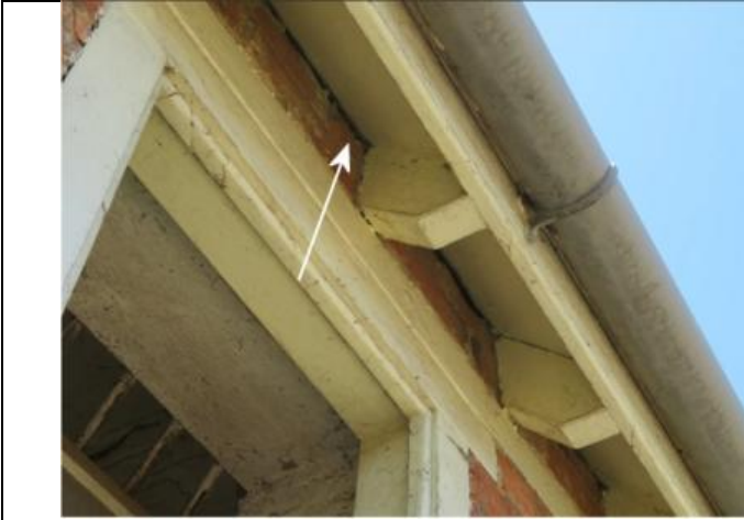
Photograph 7. Example of an opening between the soffit and the north-east wall of Building 1
