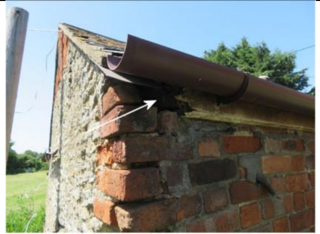
Photograph 20. Example of a gap at the corner of the wall of Building 3
