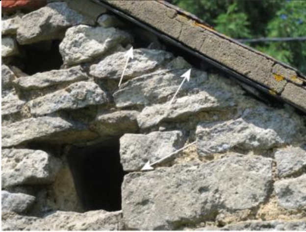
Photograph 19. Example of gaps between the roof and the south-east gable wall of Building 3
