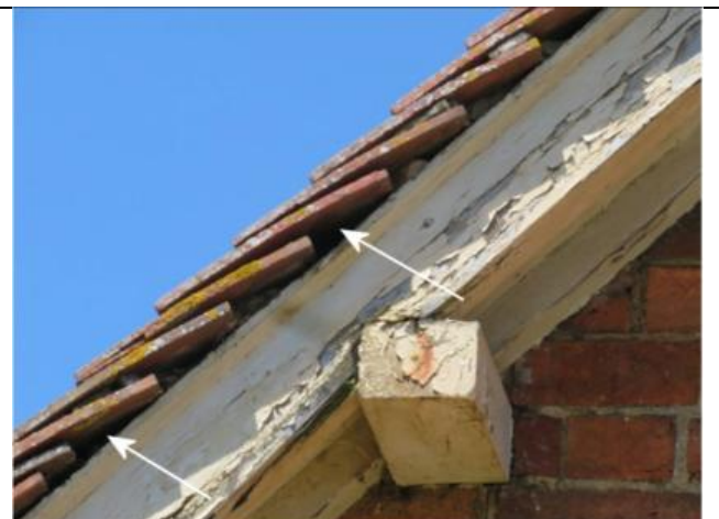
Photograph 6. Openings under tiles along the edge of the south-east gable wall of Building 1
