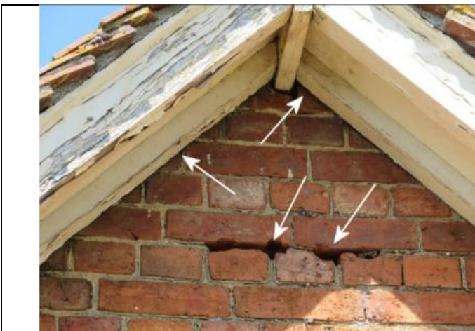
Photograph 5. Openings under the bargeboard and in the south-east gable wall of Building 1
