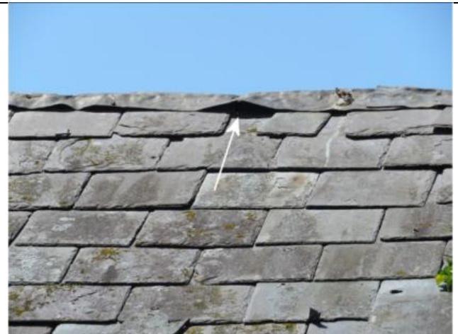
Photograph 18. Example of an opening under the lead flashing on the ridge of Building 3
