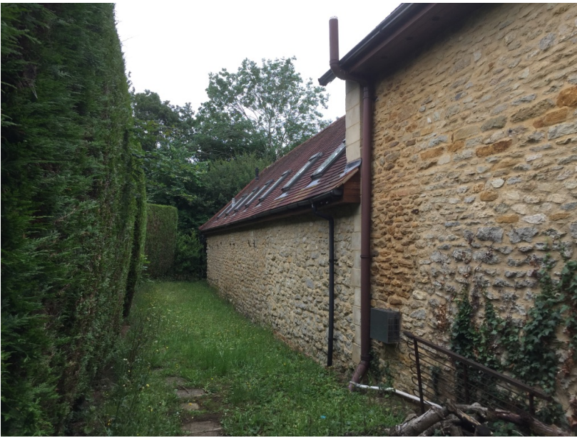
Fig. 2: Existing Rear of property (North-West Facing) with continuous 3.5m high dense Coniferous hedge-row
