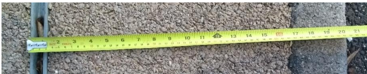
Figure 1-3: Photo of kerb to root area by 4.1 m width, measuring tape showing 0.5 metre distance
