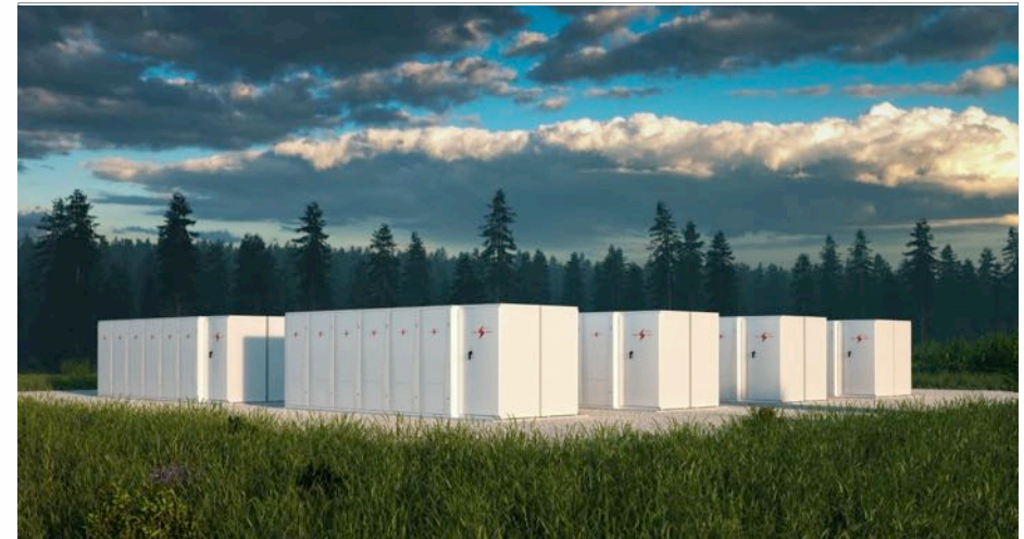
Figure 3.4.1 Utility scale battery storage: Large scale battery storage projects such as this are likely to be deployed rapidly in the coming years. They offer significant economies of scale. (© Energy Saving Trust, 2020)
