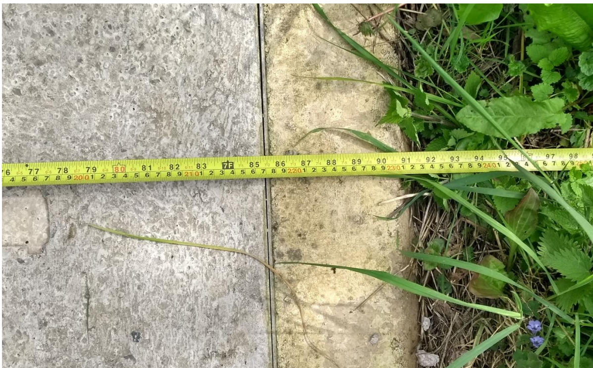
Figure 7(b): Measuring tape from Figure 7(a), other end, showing the right hand edge of the drain located within 2.20 metres from the road edge.
