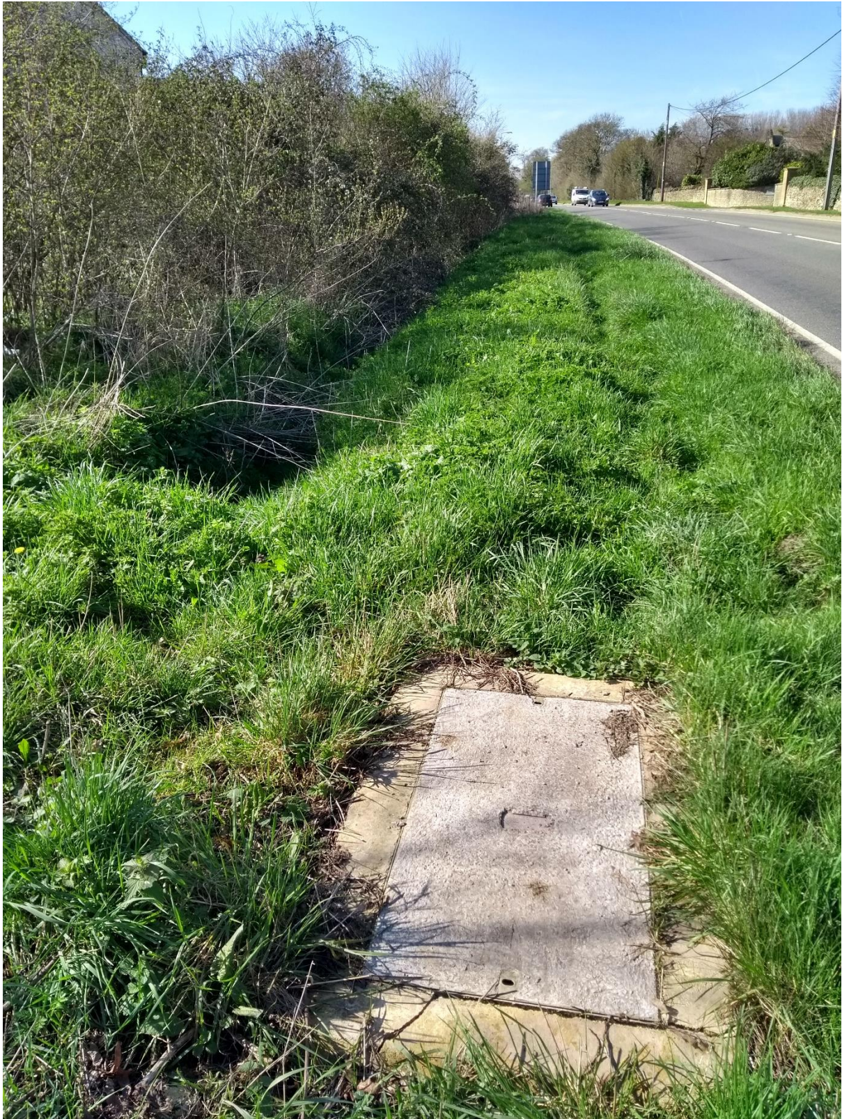
Figure 6: Closer-up view of the drain, also showing where the hedge/weeds on the left are covering the left-hand half of the sunken area.
