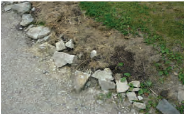
Erosion of kerbing
