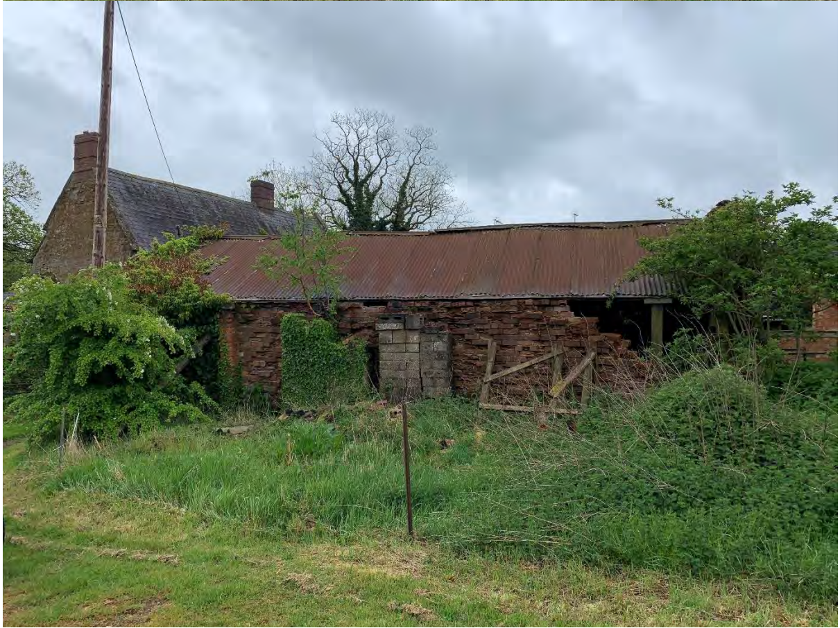
Figure 17: Buildings 7 and 8, front (top) and rear – note the very poor condition of the back wall.
