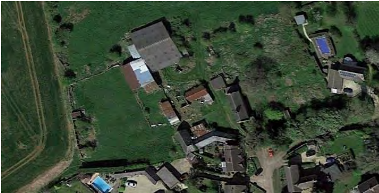
Figure 13: Google Earth images from 2009 (above) and 2017 (below) show the dramatic pace of decline in the largely abandoned outbuildings. In the earlier photograph building had lost its roof 6 in full, but only the north end of building 11 was unroofed. By 2017 its roof had gone completely, and the interior had been invaded by greenery.
