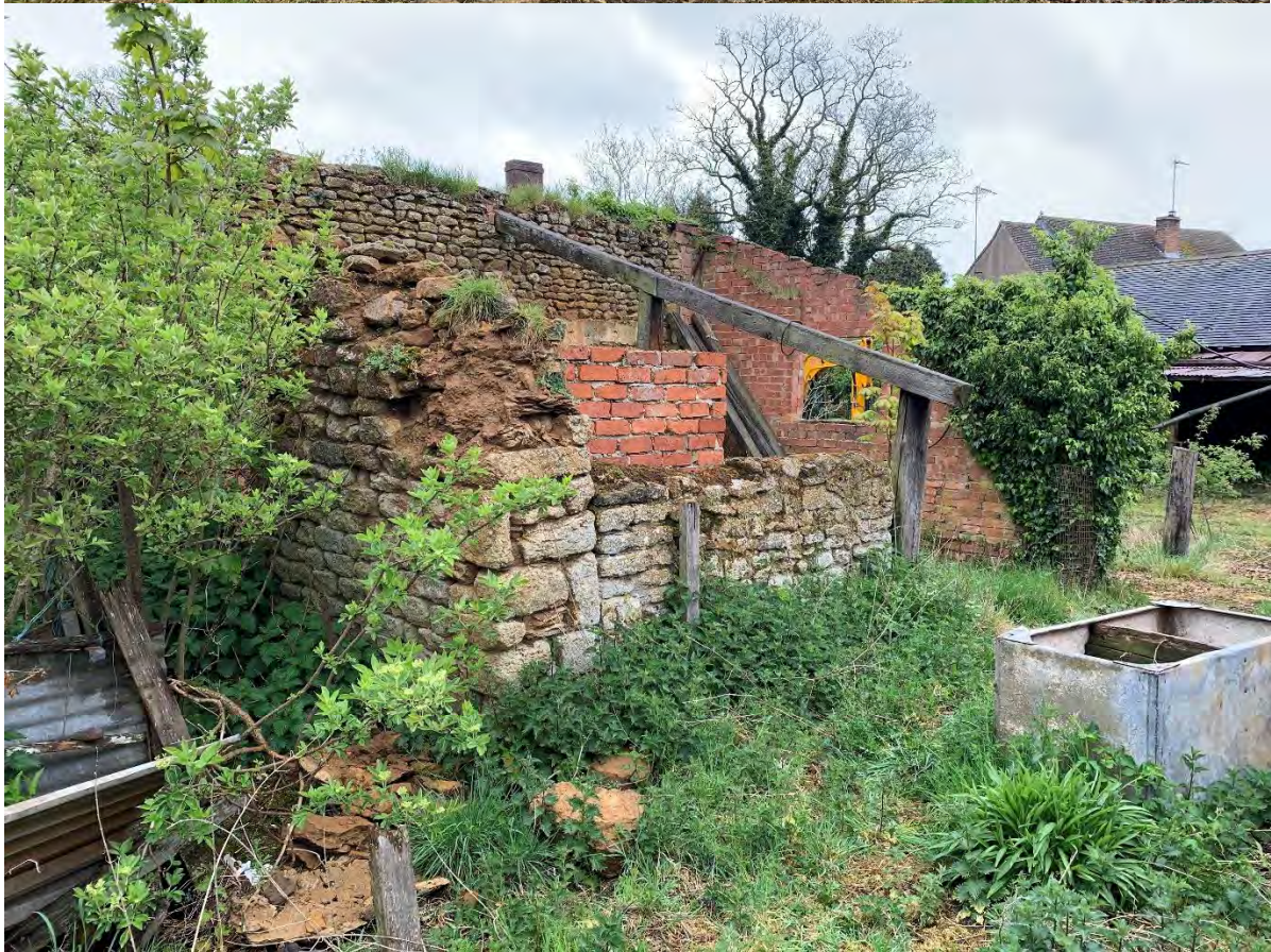
Figure 16: Buildings 5 (top, looking north-west) and 6 (looking south-east). The latter's condition has deteriorated since 2016 – compare with the same view in Soden 2016, figure 12.
