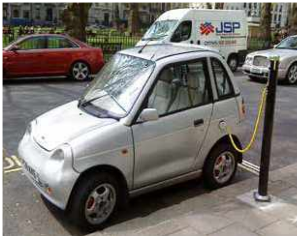
Electric vehicle charging point.
