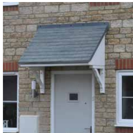
Unsuccessful example of plastic faux-tile porch, Banbury
