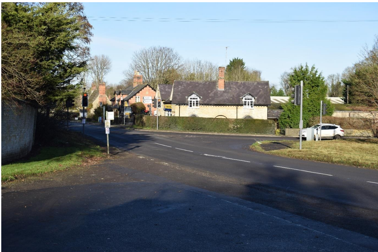
Photo 20 Middleton Stoney. Verge removed to left for footway and road widened in right verge
