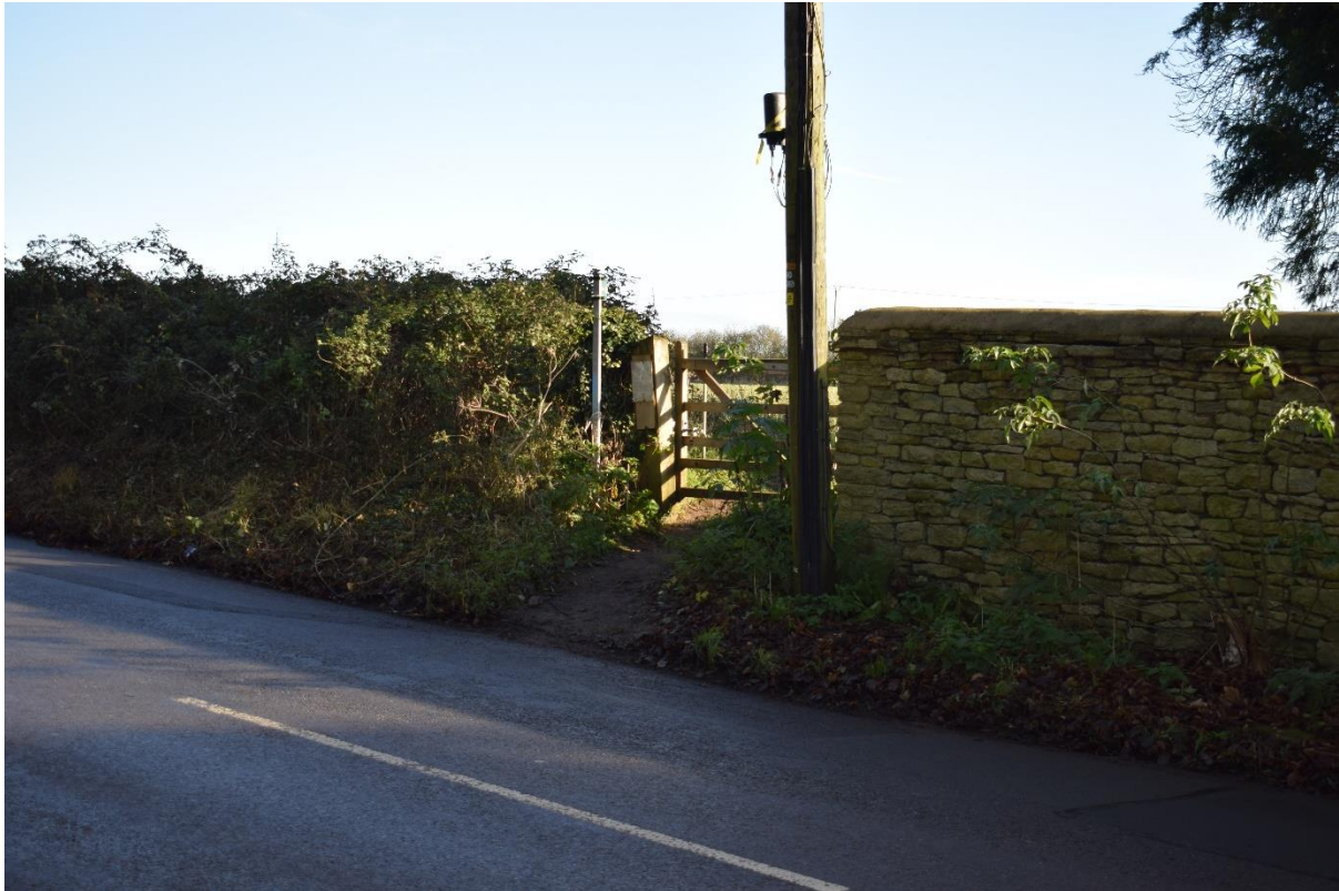
Photo 19 Kerbing, macadam and guard railing to be introduced at entrance to PROW north of Chesterton.
