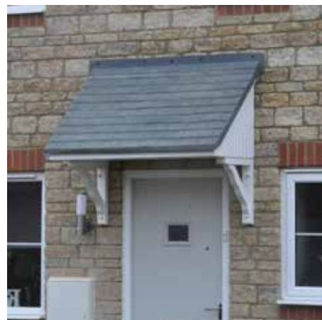
Unsuccessful example of plastic faux-tile porch, Banbury
