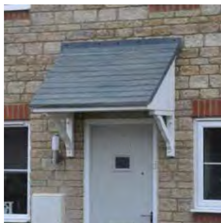
Unsuccessful example of plastic faux-tile porch, Banbury
