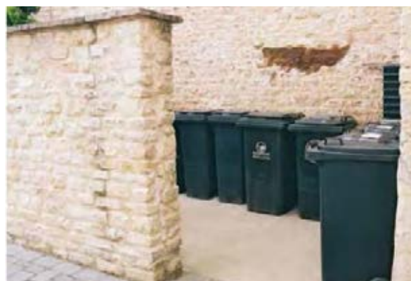
Example of an attractively designed bin store (source: West Oxfordshire Design Guide)
