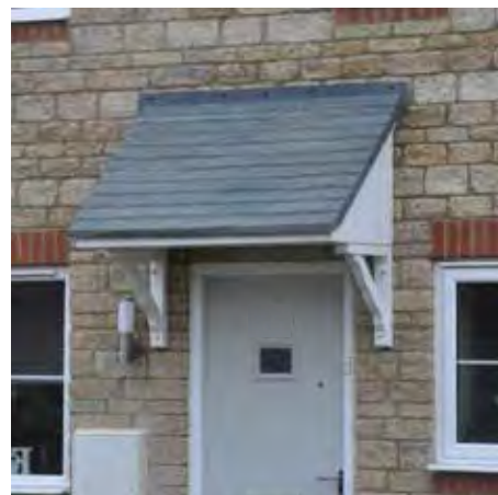
Unsuccessful example of plastic faux-tile porch, Banbury
