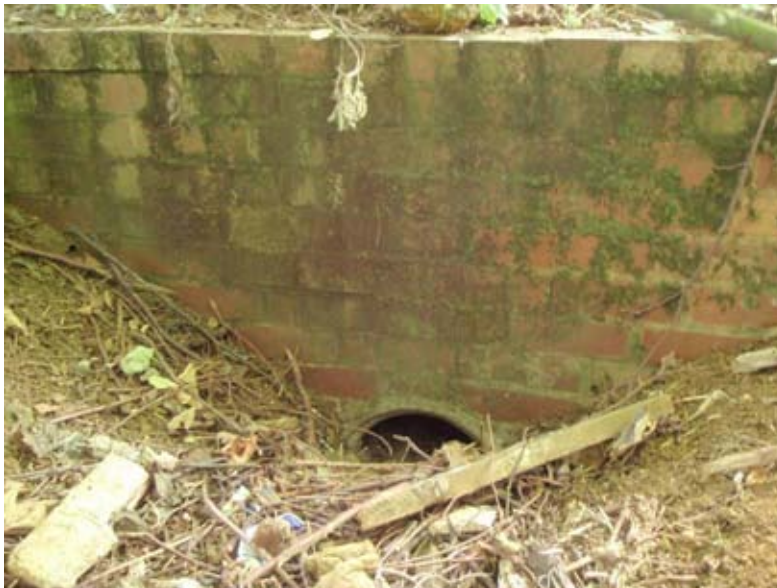
Photo 1. Brick headwall at culvert inlet on southern site boundary (field drainage ditch).
