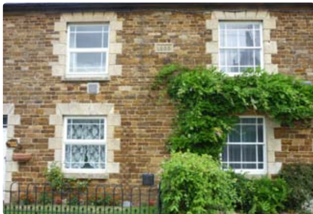
21. The heavier plastic windows to the left contrast with the slimmer and traditional timber sashes on the right
