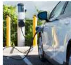
▲ Electric vehicle charging facilities
