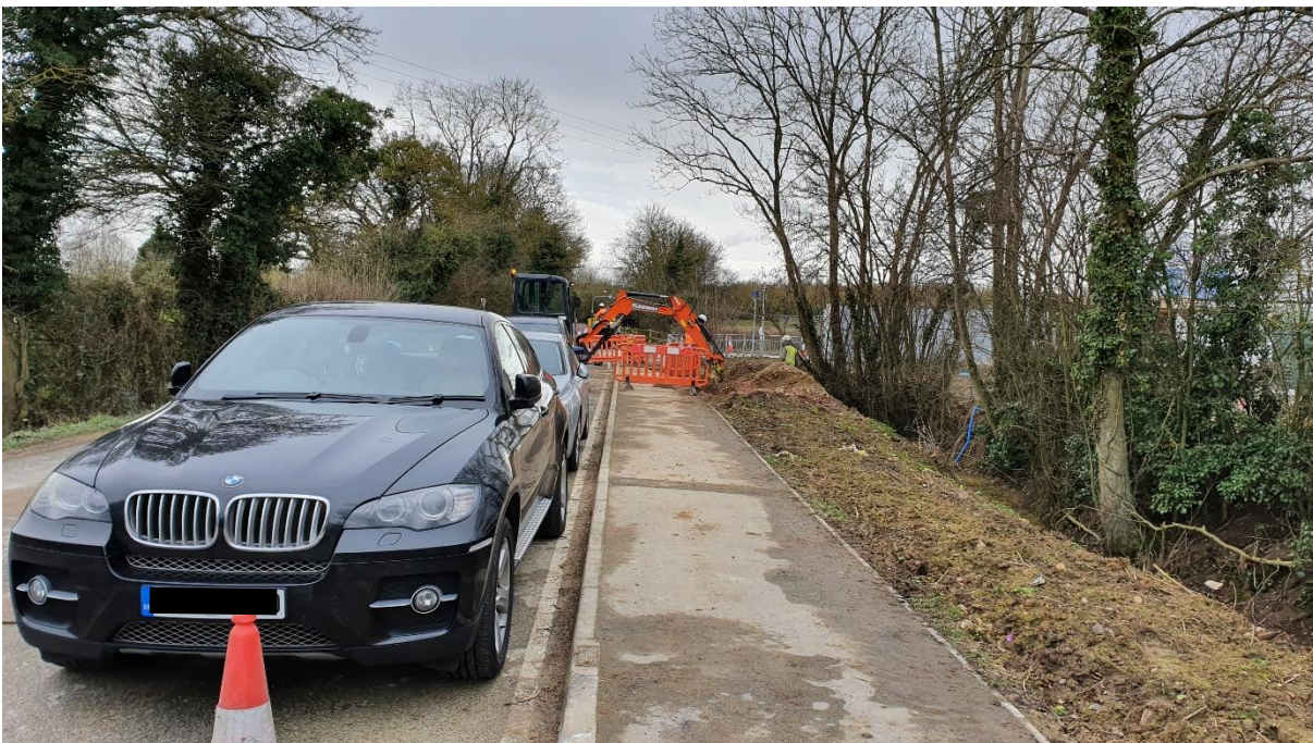
Figure 2: Existing footway / cycleway (to become footway only) on western side of Wendlebury Road.
