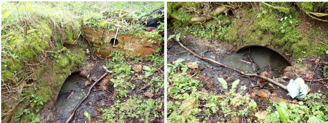
Two views of the Triangle/Frieze Way ditch with big culvert to left, set low down which takes ditch water (can be seen flowing) under Frieze Way from the Triangle ditches 29.03.2024 J A Webb photos. Brick wall to access causeway visible with pipe (no water flow). Water is backed up in ditch on the northern side of causeway but emerging from under causeway.
