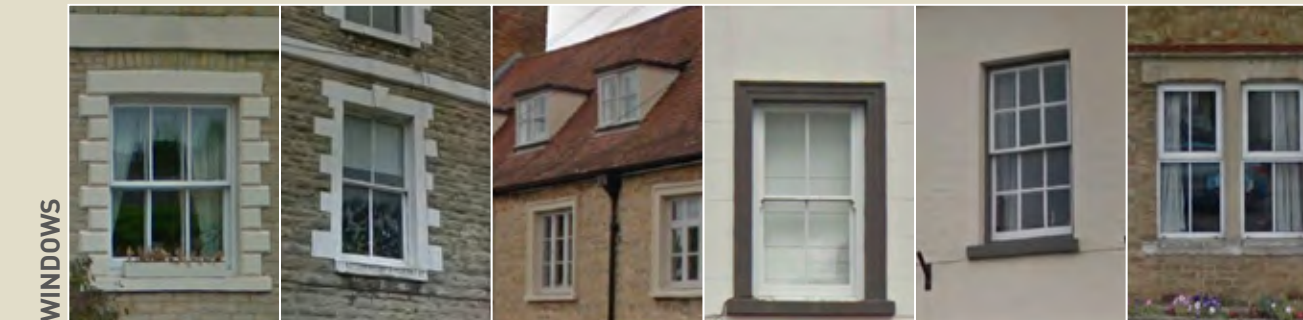
Stone header, cill and quoins. Dormer windows and solid surrounds to main windows. No header and stone cill. Stone header and stone cill.
