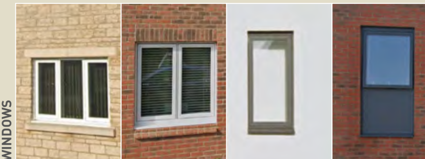
Stone header and cills. Brick header and brick cills. Contemporary style with no header or cills.
