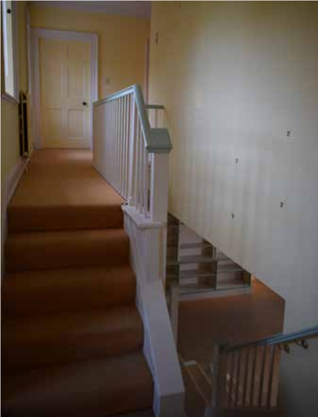
Fig 30: View of staircase first floor balustrade, with late 18th century detailing, which is considered to be original with the 1956-86 alterations. Staircase links through to the former service wing
