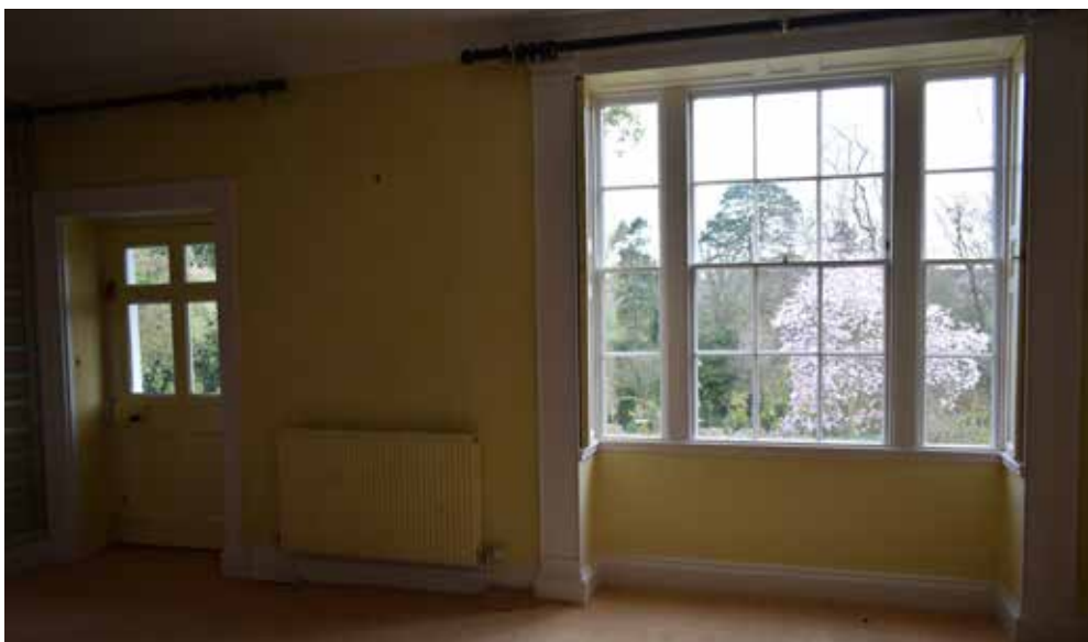
Fig 27: Reception hall looking south showing back door which was originally within a separate hall (wall removed in the 1956-1986 period) with the tripartite windows and pilasters. Cornice details still survive in both rooms
