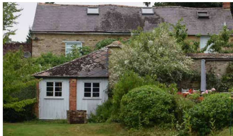
Fig 25: View looking west from the garden showing the rear brick wall and brick piers with timber infilling of two bays.
