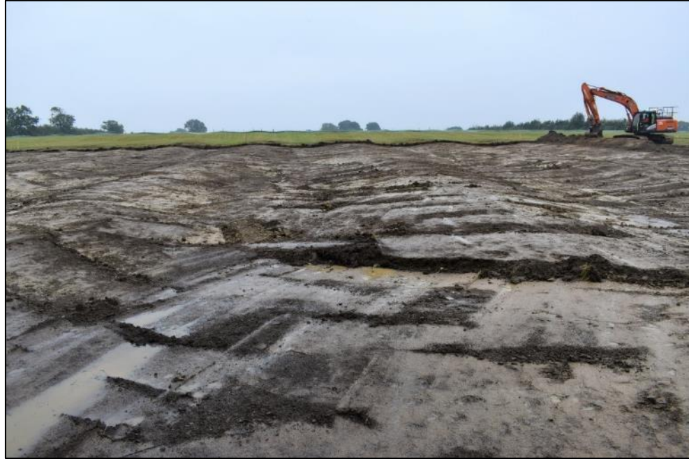
Plate 15: View of ridge and furrow during topsoil strip in northern area of the Site, looking south-east
