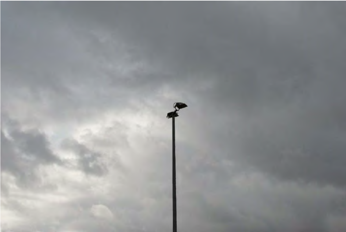
Figure 5.1: Sports lighting luminaires used at Stratfield Brake Sports Ground. Twin head arrangement.
