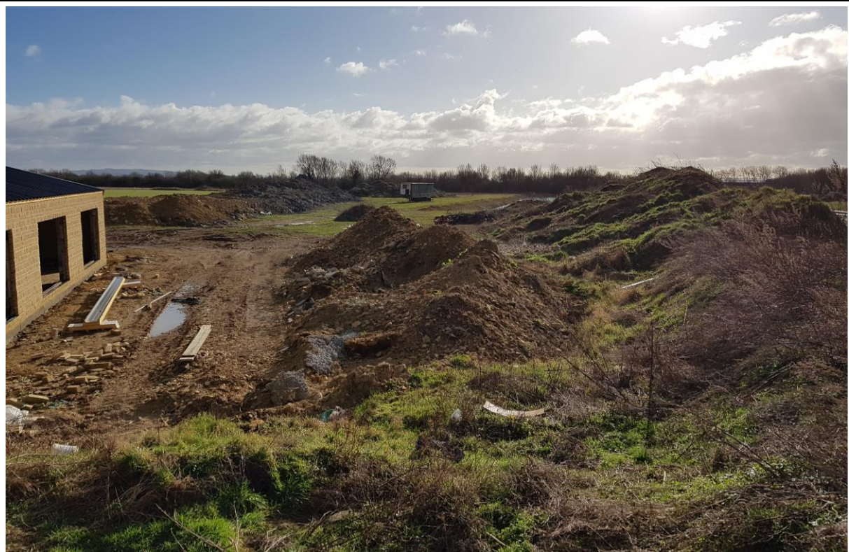
Photo 17: View south along the western boundary of material stockpiles, with a recently constructed building in the foreground.
