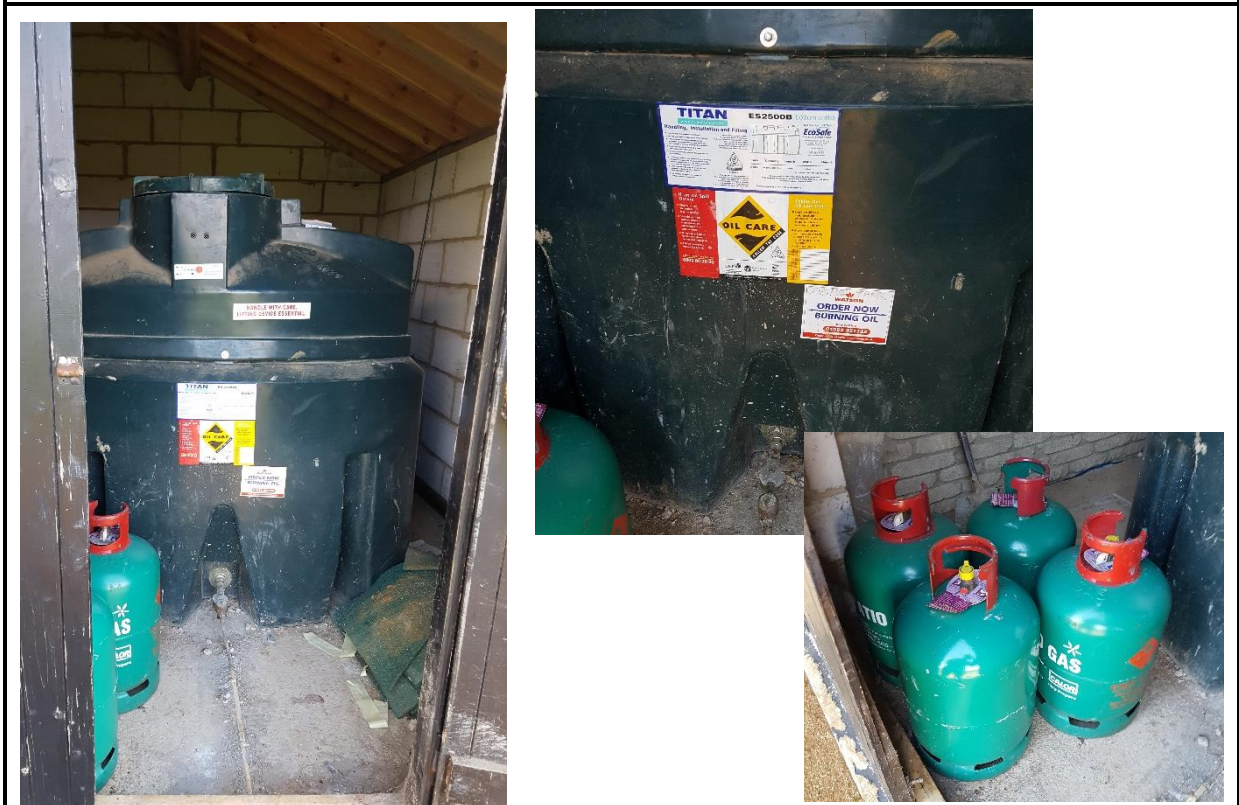
Photo 12: Bunded tank and gas bottles located in the south-west corner of the clubhouse buildings
