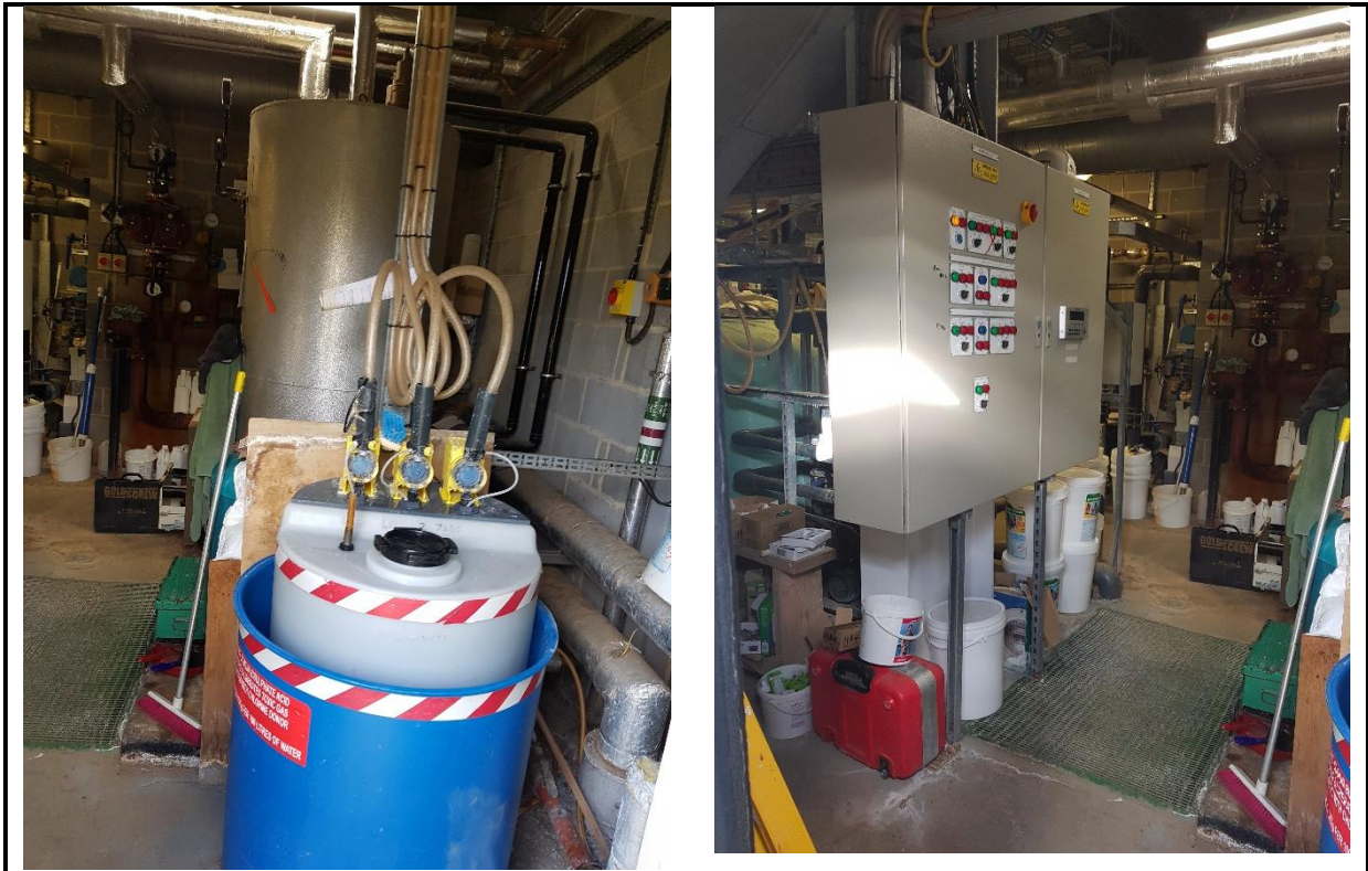
Photo 11: Plant room located in the south-east corner of the clubhouse buildings
