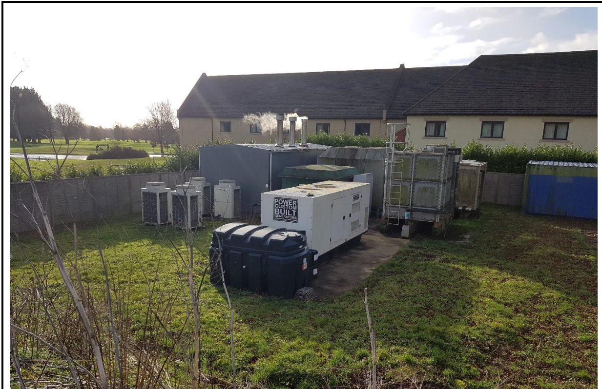
Photo 5: View of the air conditioning units, bunded oil tank, generator, electricity substation, gas house and water tanks immediately north of the clubhouse
