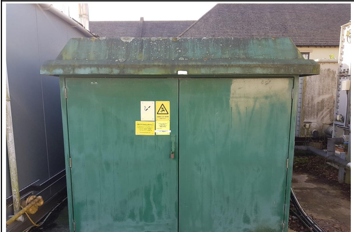
Photo 8: View of the electricity substation immediately north of the clubhouse
