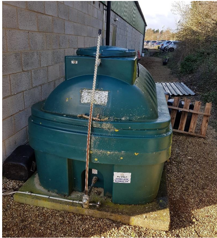
Photo 13: Bunded oil tank located immediately north of the maintenance building
