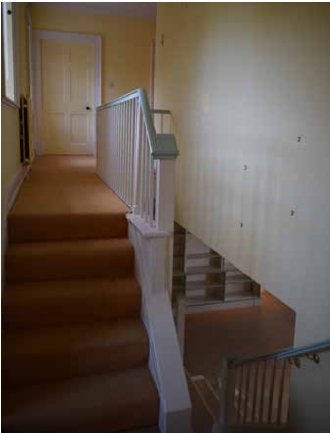
Fig 32: View of staircase first floor balustrade, with late 18th century detailing, which is considered to be original with the 1956-86 alterations. Staircase links through to the former service wing
