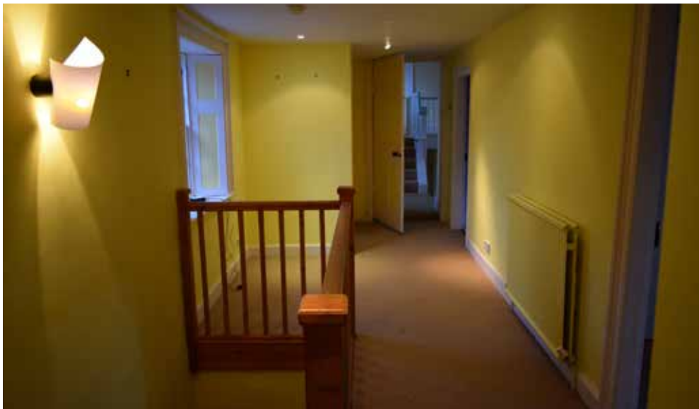
Fig A3.7: Balustrade of the current stair (recent) removed and new balustrade installed. Door to the current bedroom adjacent to the door opening from the main range to be moved to remove conflict with this door
