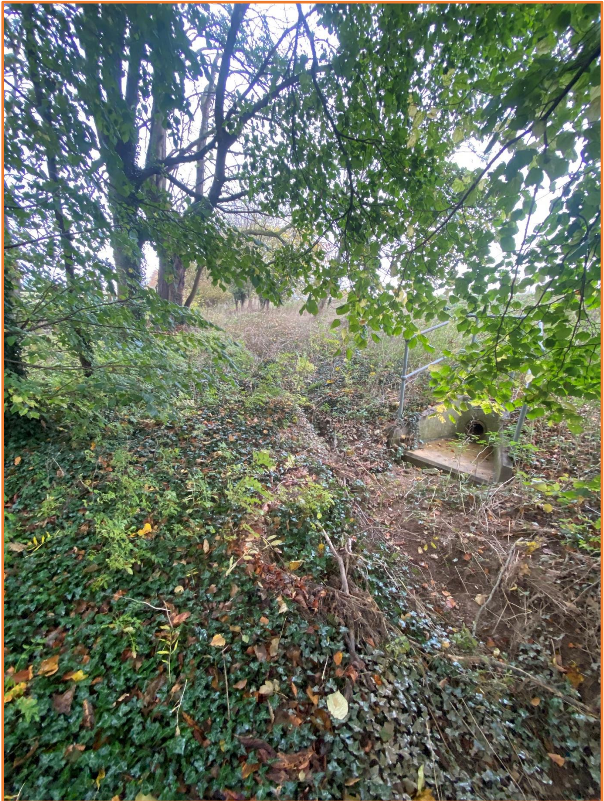
Figure 8: Ditch downstream of the site prior to being culverted beneath Bloxham Road, and phase 2 outfall headwall
