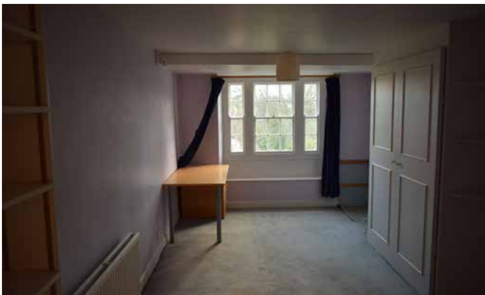
Fig 37: The bedroom which is proposed to be adapted to an ensuite showing the c. 1930 extension, marked by the ceiling beam, and the tripartite window which matches those of the garden elevation of the main range
