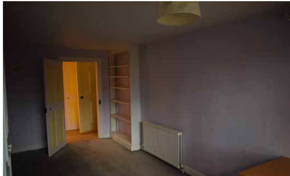
Fig 38: The adjoining bedroom looking towards the eastern wall which it is proposed to open up to create access to the ensuite
