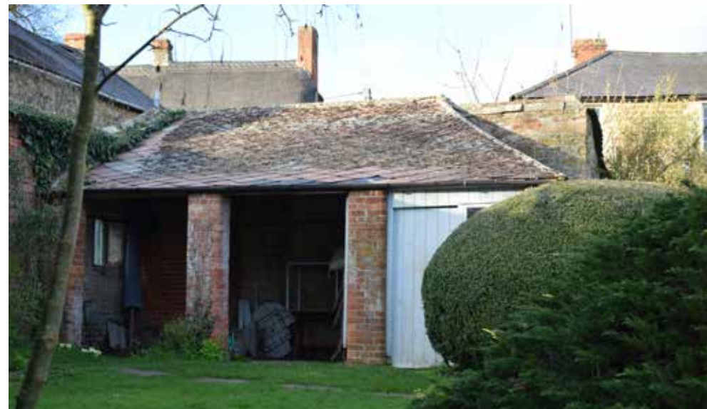
Fig 26: View of the potting shed from the garden looking north showing three sections divided by brick piers with the eastern section enclosed and the hipped roof. The gable roof sits against a brick wall which has a door and a window into the end bay
