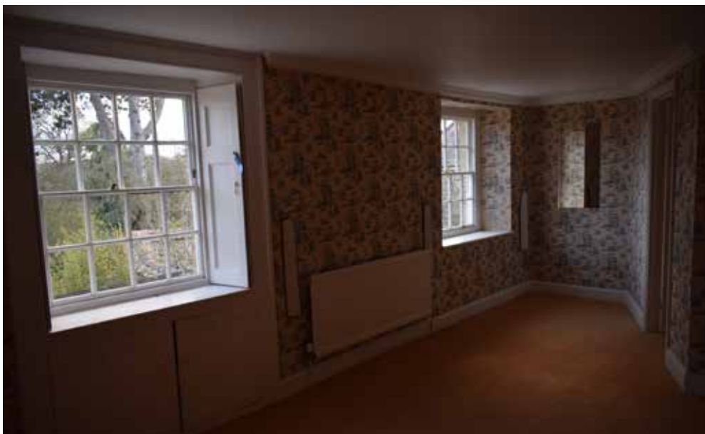
Fig A3.8: Bedroom in former service wing with ensuite inserted. Proposal involves the removal of the ensuite and installation of a non-structural dividing wall to create two bedrooms
