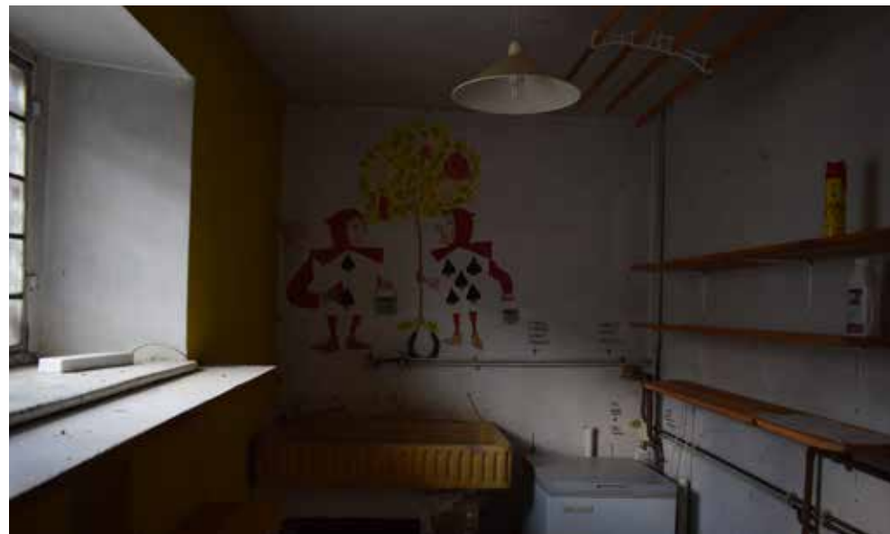
Fig A3.5: Boiler room which is proposed to be combined with the utility room adjoining with access via the existing door
