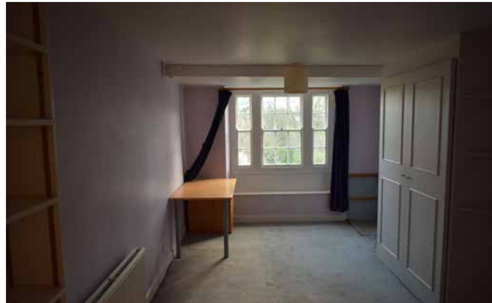
Fig A3.9: Small box room extended c. 1930s by a lean-to extension over a ground floor bay window. Original size of the room marked by encased ceiling beam.
