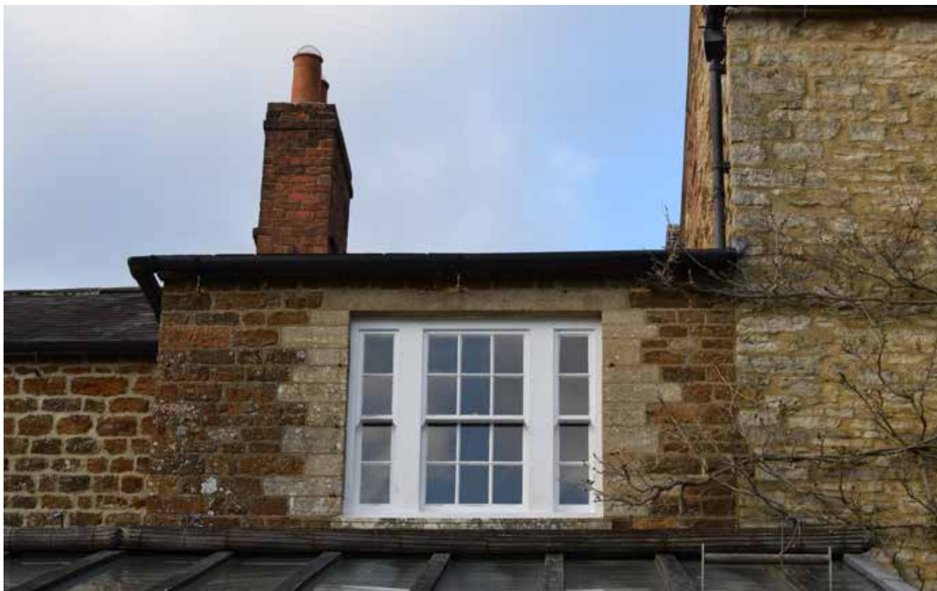
Fig 37: Close up of the tripartite window on the rear (south) elevation of Cedar Lodge for the small box bedroom illustrating the external 'gentrification' of this part of the building to match the window pattern of the main range
