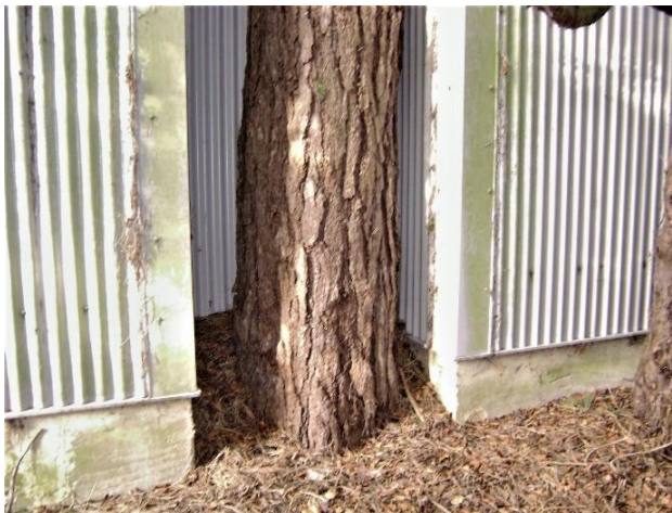
Photograph 13 – Pine tree T76 with the stem enclosed on three sides by the concrete base of the building.
