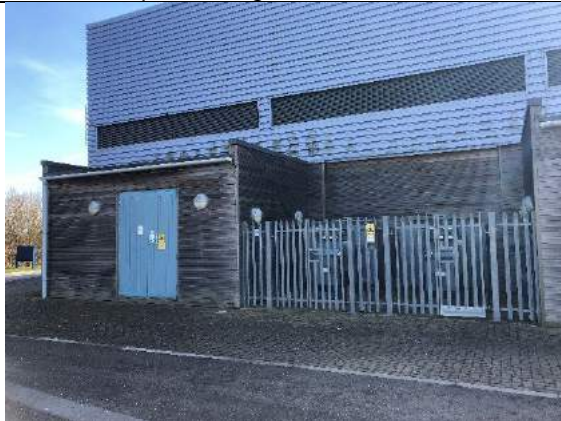
Plate 9: Transformers at rear of main facility
