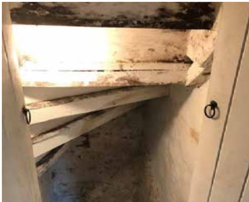
Existing Timber Stairs from below, the black mould from damp ingress into the existing stairs will need to be addressed or removed if the timber is completely rotten.
