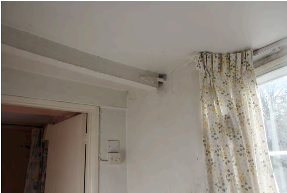
Photo showing the beam to the kitchen ceiling affected by the wall leaning outward
