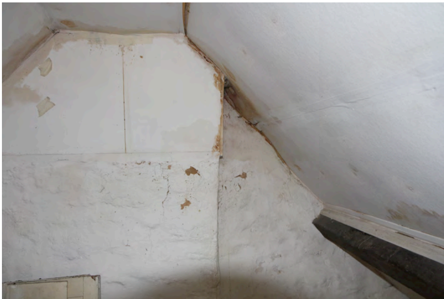
Photo showing the damage ingress to the north gable
