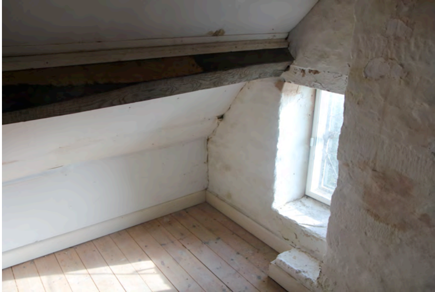
Photo showing the damp ingress to the south gable
