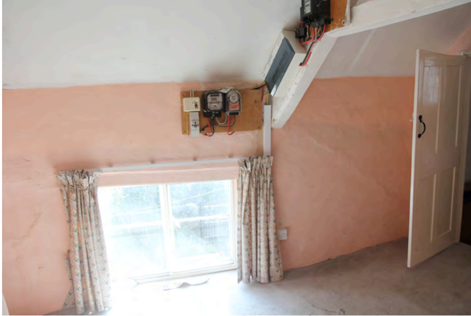
Photo showing the electrical incoming mains and distribution boards
