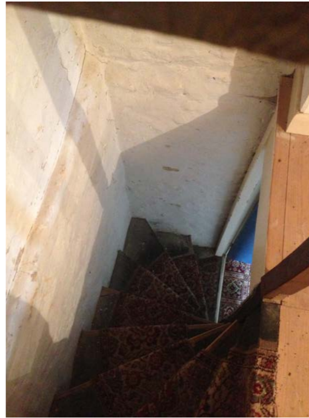
Existing steep winder staircase
